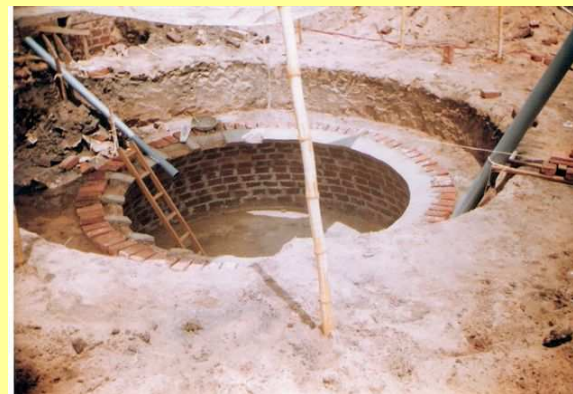
CoBu develops biogas digester as a tool of sustainable sanitation, Malinyi, Tanzania
