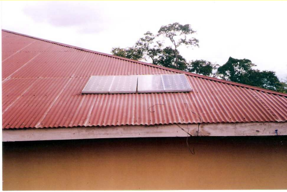
360W Solar Generator at Mbingu Sisters Centre-Tanzania, installed on the roof without frame. CoBu improved the installation by developing a 1m high metal frame
