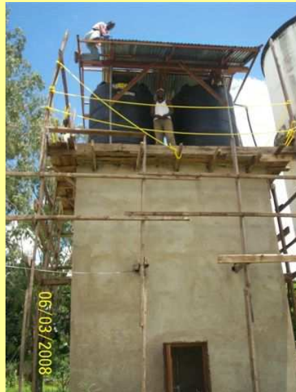
10,000 ltrs tank at Lugala Lutheran Hospital, Tanzania, planned and developed by CoBu
