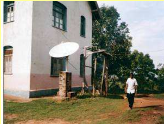
Panels installed East-West orientations. CoBu improved installations at Itete Catholic Parish, Tanzania.
