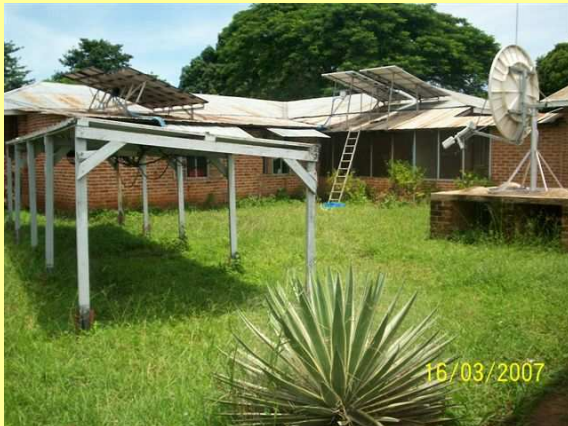
CoBu participated in the development of 6Kw solar generator at Lugala Lutheran Hospital, Tanzania.
