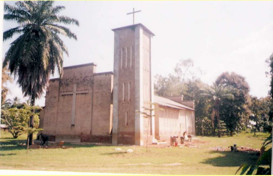
CoBu carries out the rural structural renovation works. St. Pius X Parish Church, Malinyi, Tanzania.
