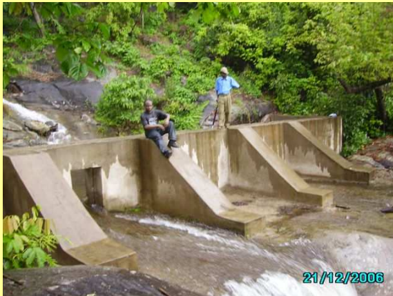
CoBu plans, designs and gives technical supports in the water supply projects. In the picture, intake structure for gravity water supply at Chita village in Tanzania.
